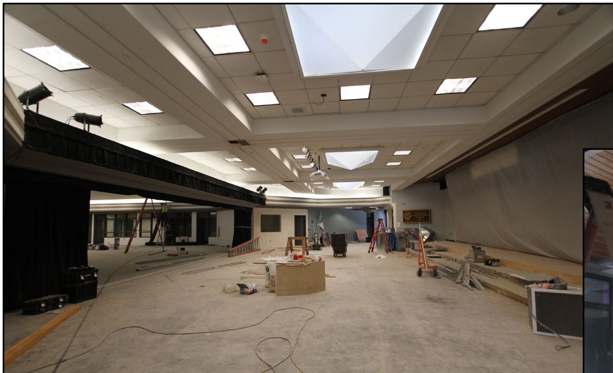
New control booth in Multipurpose Room
