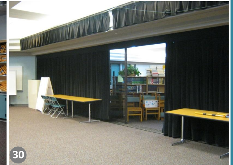
Sliding glass partition between MPR and Library
